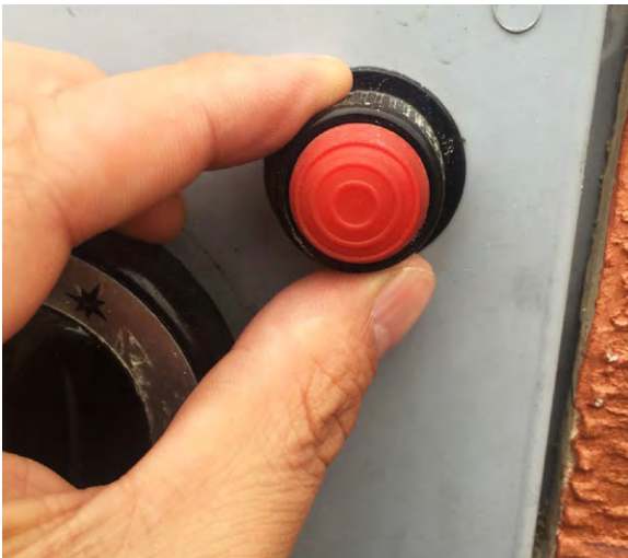
Photo 1 Remove dead battery.
